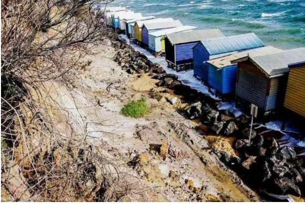
MM North sheds with sea flowing under. Boulders dumped at cliff toe and “sculpting” of cliff face, long since proven futile. November 2019 © Keith Platt.
